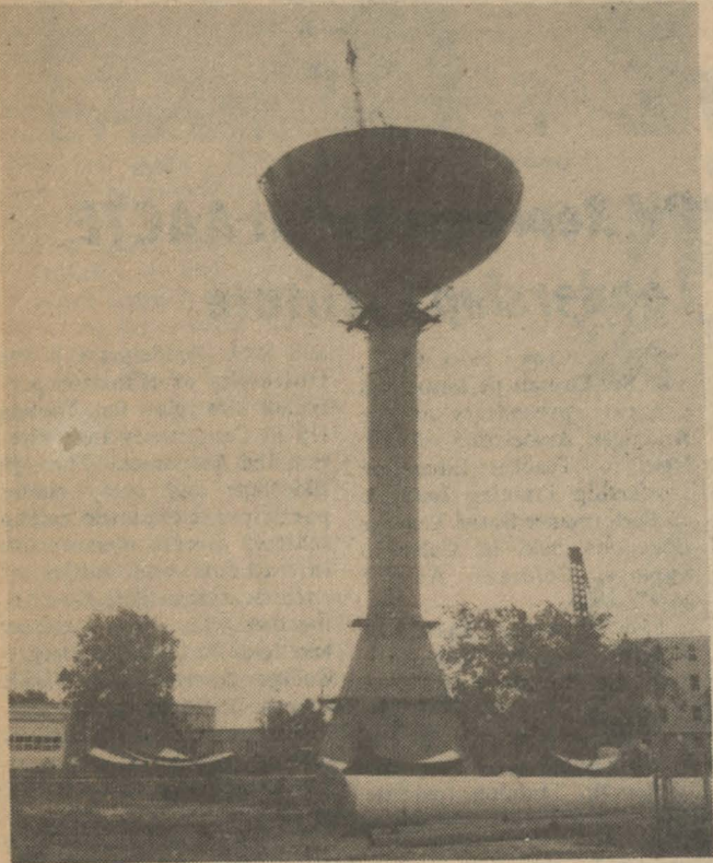
GIANT HIGHBALL? Wrong again. But the new water tower going up on campus looks much like a huge cocktail glass. The daring construction is providing PV residents with plenty to watch and leaves much for the imagination.
