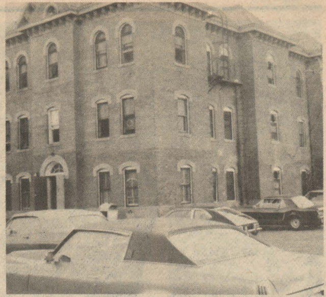
OLDEST CAMPUS STRUCTURE COMING DOWN — Foster Hall, erected in 1894 is being demolished along with Luckie and Minor Halls and several other buildings and cottages. Renovation and repair work is progressing throughout the campus, while plans for new construction are underway.
