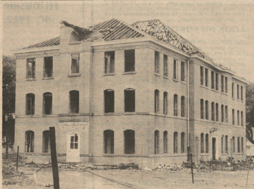
A HEAP OF PV HISTORY — Thousands of grads and ex-students, male and female, made Luckie Hall their home during college careers. Now it is being demolished — making way for newer and more modern facilities. Built in 1912, the dormitory was named for Professor C. W. Luckie (1898-1909).
