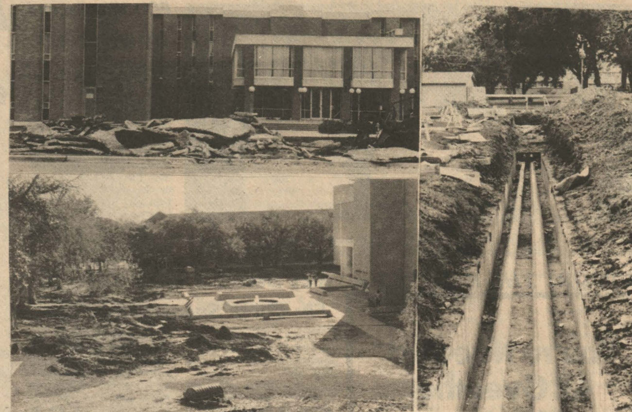
CAMPUS CONSTRUCTION — Much of the central campus is now undergoing a facial change — now ugly, but with promise of beauty in months to come.
