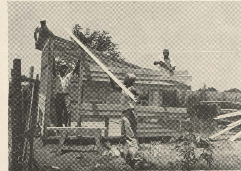
AGRICULTURAL ENGINEERING STUDENTS CONTRIBUTE TO PRAIRIE VIEW'S EXPANSION PROGRAM —Students in farm building construction class are shown in the photo above erecting a shed for beef cattle on the college farm. Purlins are being placed by E. B. Johnson and Jake Cleveland; corner posts are being braced by Verbe Norman and Norman Barlow. The group in the lower picture is completing a poultry house for one of the college residences. Clyde Wedgeworth and Garland Washington are putting on roof sheathing; Claude Jones is measuring the door opening; and Lennie Lyons is sawing-off side boards.
