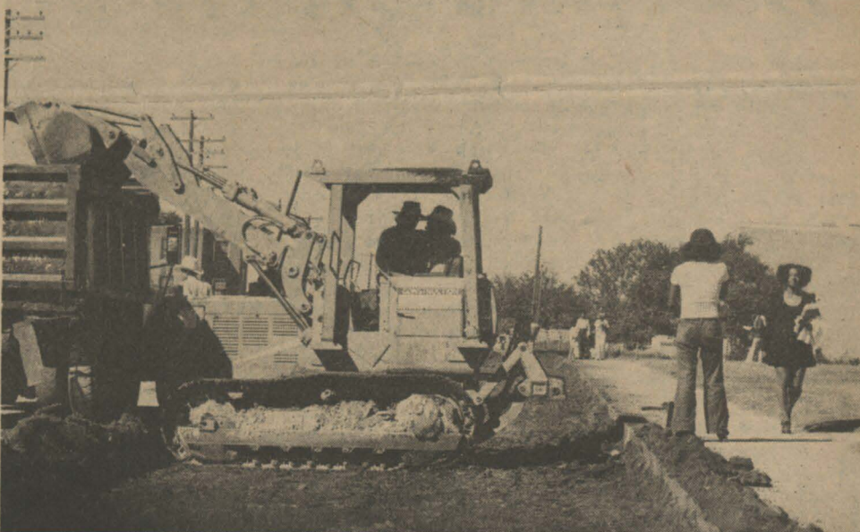
ROAD REPAIR — Campus streets expected soon. The campus By-Pass are getting much needed repair. Completion of work which has hindered borders of the campus, is also in final auto movement across campus, is stages.
