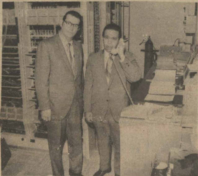
FIRST TELEPHONE CALL — President A. I. Thomas is shown making the first official telephone call on the new Centrex installation at Prairie View. Bell Telephone official Mr. Gene Brown is pictured with Dr. Thomas in the Company's headquarters near City Hall.
