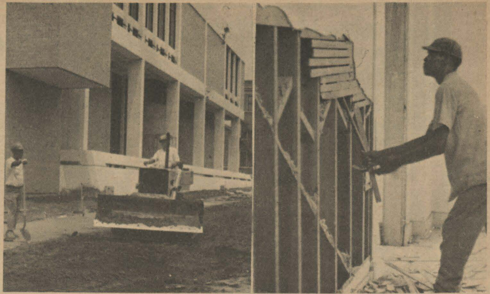
CONSTRUCTION PROJECTS (at left) and demolition of older structures. UNDERWAY ON CAMPUS — Landscaping ground completed building
