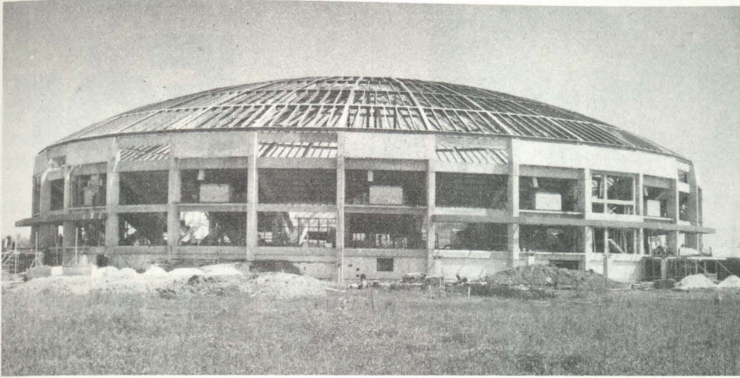
The $9 Million Dollar Domed Stadium currently under construction will bring to the campus many road shows, while being used for basketball and special assemblies.
