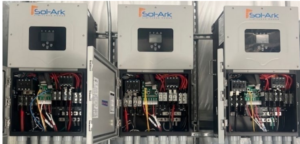
Fig. 98 Sol-Ark 3-Phase Wiring Configuration for the Platform [181].
