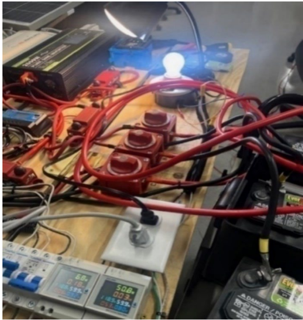
Fig. 73 Prototype Components: CT's, DC Switches, MPPT, and Inverters.
