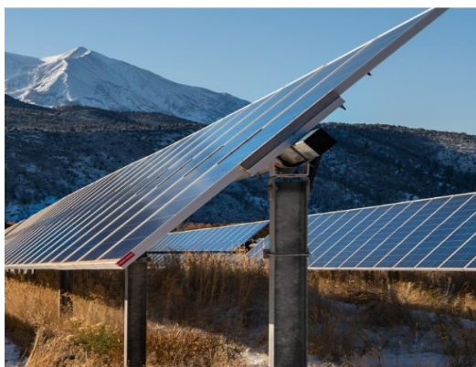
Fig. 91 Fixed PV Degree Installation [170].
