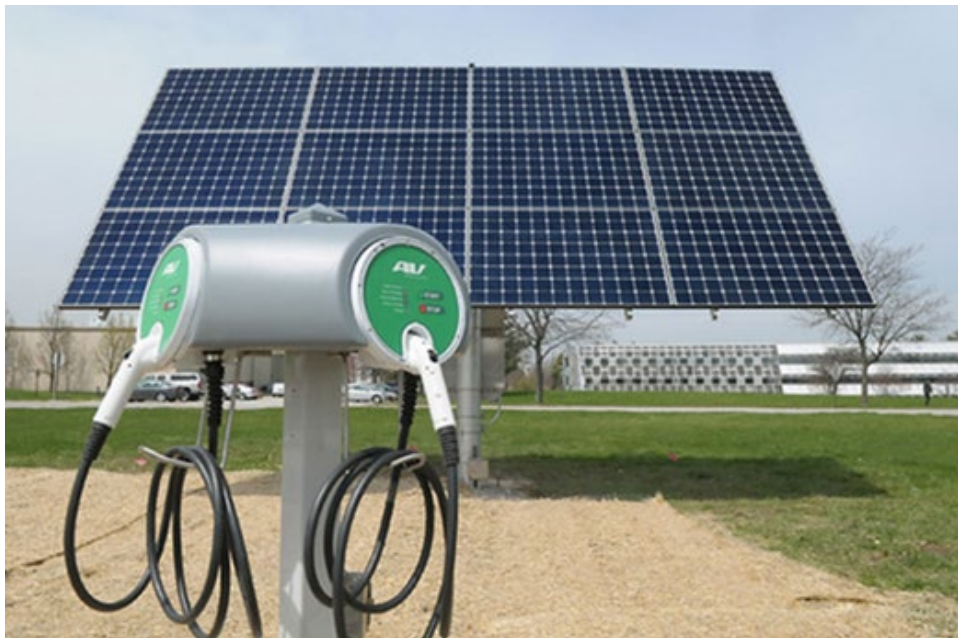
Fig. 28 PV Solar Charging Stations [66].
